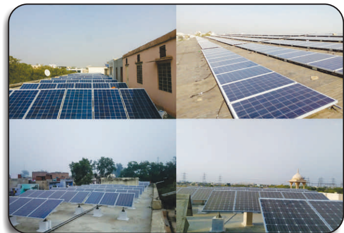
Solar Power plants at discrete locations across Rajasthan under RREC Rooftop programme
