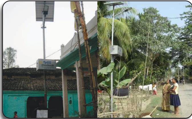
HLS and SLS Systems installed under CSR of Customer
